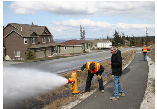
Monitoring flow tests and pressures
